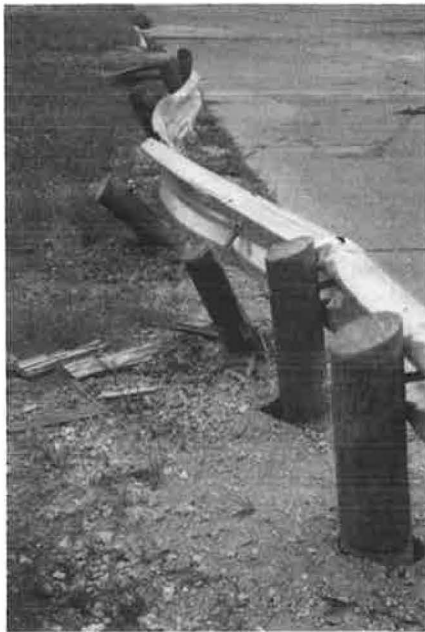
FIGURE 16 Barrier damage after Test 3.
