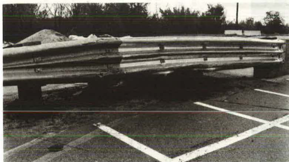
FIGURE 12 Photographs of test No. 4 guardrail damage.
