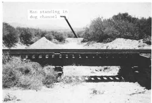
FIGURE 12 View looking downstream at railroad bridge in south Benson, Arizona. The opening was completely filled during a 1-hour flash flood on July 6, 1981. Note the depth of the channel where the filled material has been removed about 100 yards downstream from the bridge. See figure 11 for location of photograph.
