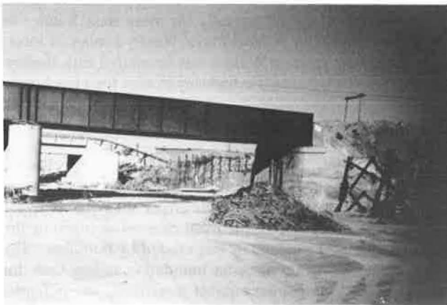
FIGURE 7 View looking downstream at the right bank of Rillito Creek at the Southern Pacific and Interstate 10 bridges at Tucson, Arizona. The failure of the wire-rock revetment at the abutments is typical for base-level streams in the area.
