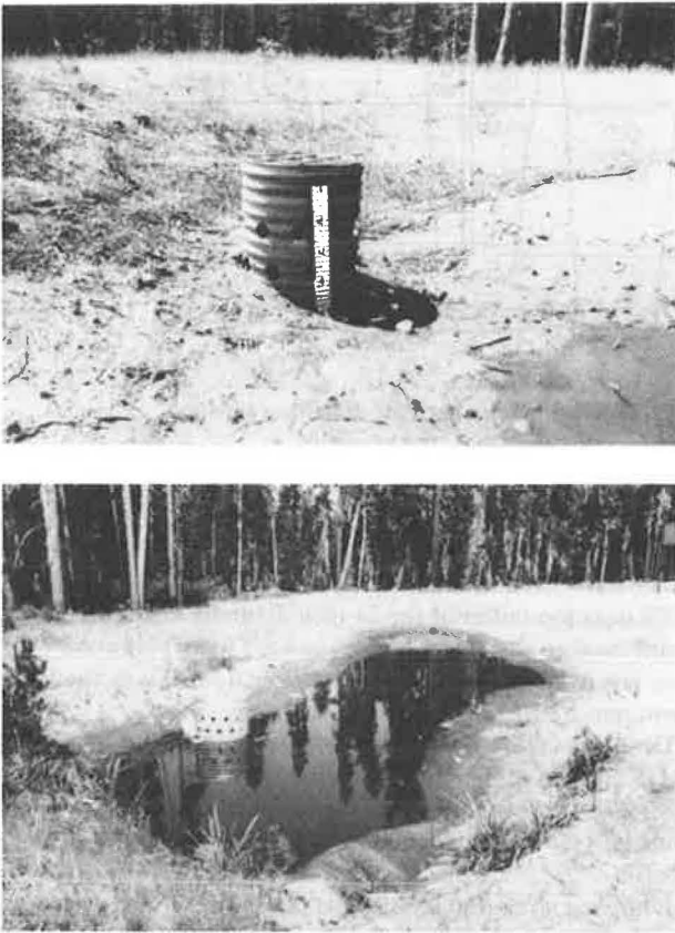
FIGURE 7 (Top) Outlet pipe riser in upper basin. (Bottom) Outline pipe riser in lower basin.
