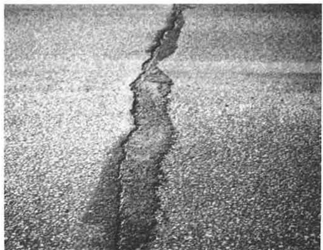
FIGURE 4 Spray patch of crack with emulsion and sand aggregate—crack remains unsealed.
