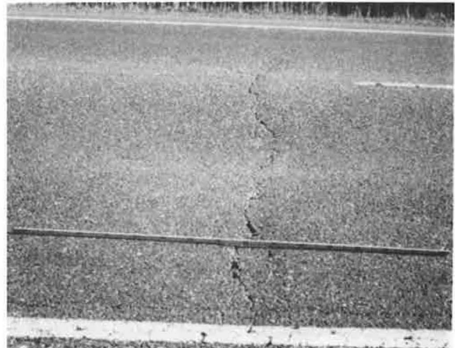
FIGURE 3 Cupping of transverse crack in summer.
