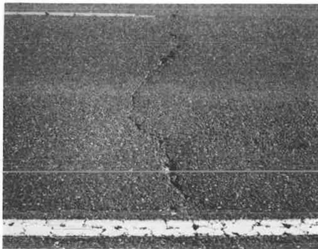
FIGURE 13 Unsealed transverse crack develops multiple cracking and spalling on Highway 17, control section.
