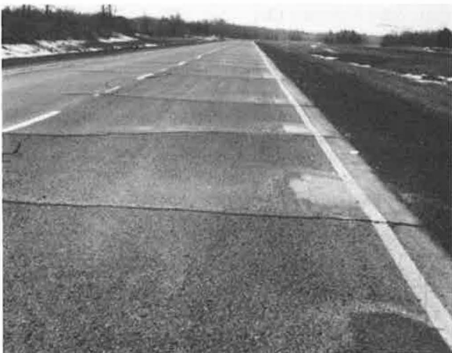
FIGURE 2 Lipping of transverse cracks in winter.
