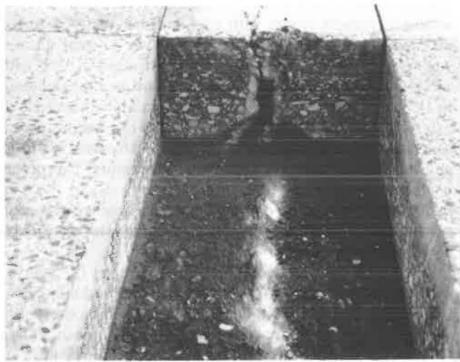
FIGURE 12 Unsealed transverse crack deterioration continues upward unchecked on Highway 17, control section.
