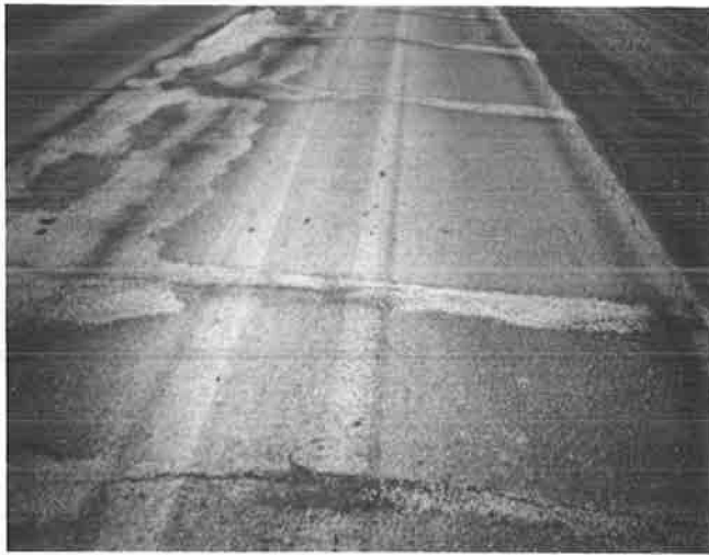
FIGURE 5 Spray patch of cracks with emulsion and sand aggregate—created small ridges at cracks that are detrimental to rideability.
