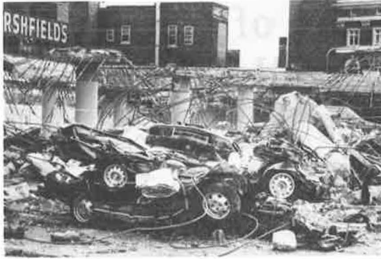
FIGURE 2 Collapse of a Minnesota parking garage due to corrosion of reinforcing steel (15).
