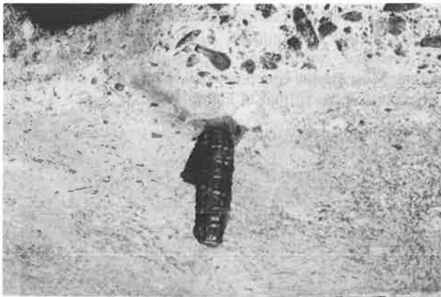
FIGURE 19 Corroded reinforcing steel stud protruding from concrete at Humboldt Harbor breakwater (July 1988).
