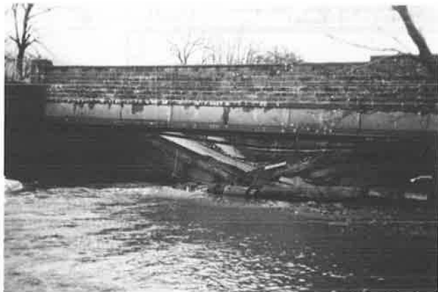
FIGURE 2 Ynys-y-Gwas bridge after collapse (photographs courtesy West Glamorgan County Council).
