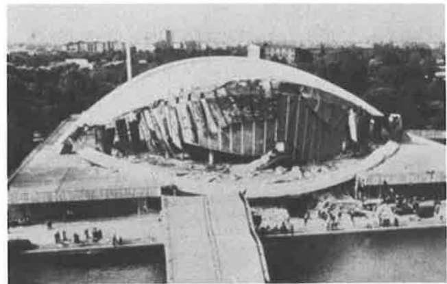
FIGURE 1 Collapse of the Berlin Congress Hall due to hydrogen-assisted cracking of post-tensioning cable.
