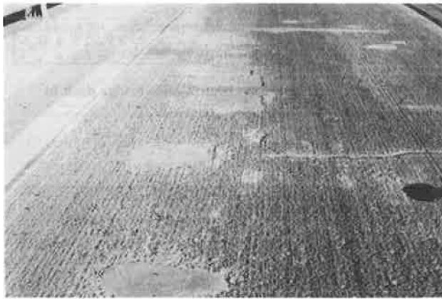
FIGURE 11 Spalling pattern on bridge under repair on I-90 in central Washington State (September 1986).
