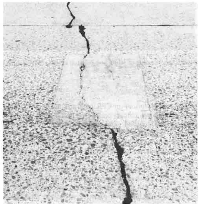
FIGURE 8 Performance problems of shallow-depth patches. (top) Cracking and breakup of shallow-depth patch adjacent to crack. (bottom) Cracking through a partial-depth patch.
