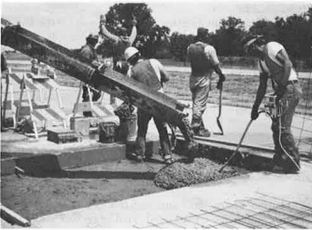
FIGURE 3 Construction of doweled full-depth patches. (top) Drilling dowel holes for doweled full-depth patch. (bottom) Pouring concrete in doweled full-depth patch.
