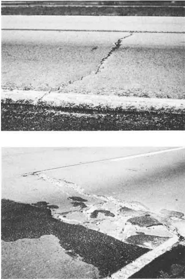
FIGURE 1 Major distresses noted on I-65 portion under study. (top) Faulted crack. (bottom) Broken-up slab.
