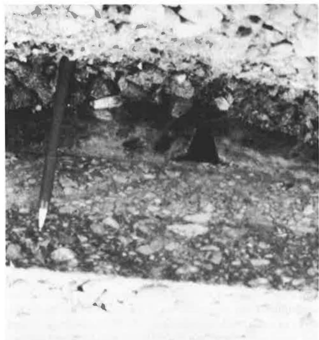
FIGURE 8 Cut-away section of asphalt overlay over a PCC pavement joint (ballpoint pen shows scale).
