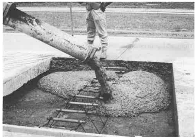
FIGURE 4 Construction of inverted T full-depth patches. (top) Excavation for full-depth inverted “T” patch. (bottom) Pouring concrete for inverted “T,” full-depth joint replacement patch.
