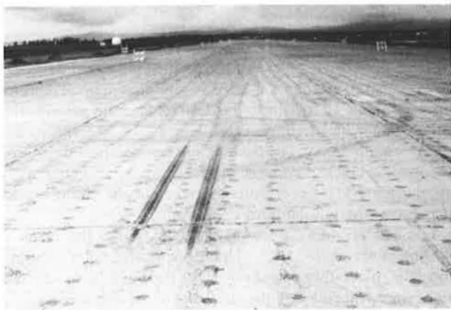
FIGURE 5 Overall view of cracking pattern.
