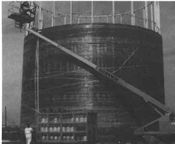
FIGURE 9 Fabricating a 42-ft-diameter composite structure on the job site by process of twine winding.
