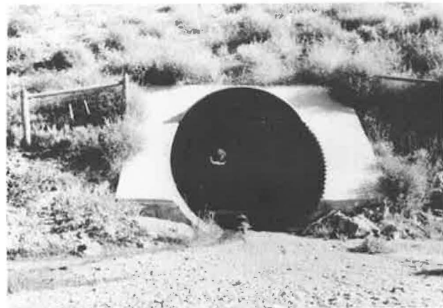
FIGURE 24 Pipe inlet at Spring Creek installation.
