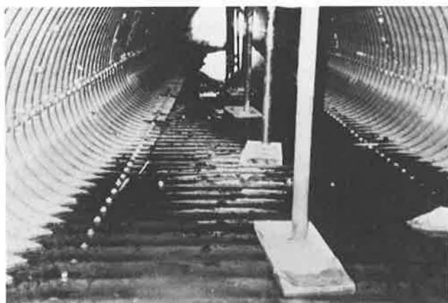
FIGURE 3 Uplifting of bottom plates in pipe arch structure.
