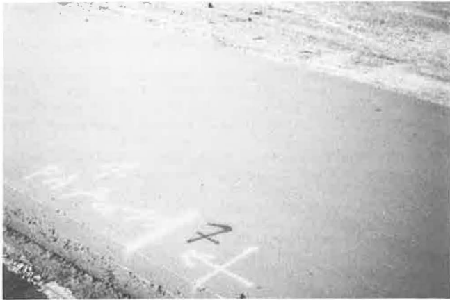
FIGURE 15 Construction of slab. Note sealed appearance of upper surface and straightness of slab edge. Maximum thickness laid was 32 m.
