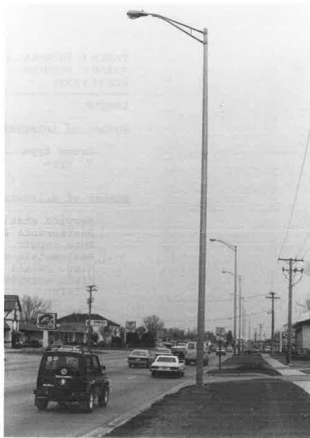
FIGURE 3 Typical view of Ogden lighting unit.
