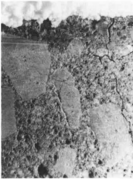
FIGURE 15 Cracks in a silane “sealed” concrete cup that occurred during the first cycle of salt water treatment. The silane did not keep salt water from moving through many limestone aggregates. The cracks go through some aggregates and alongside others.
