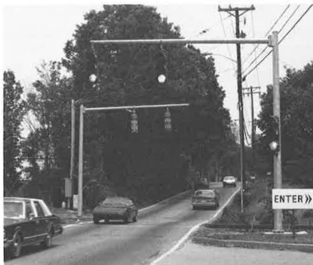
FIGURE 10 Highway traffic signal system installed at Cedar Drive crossing in Knoxville, Tennessee.
