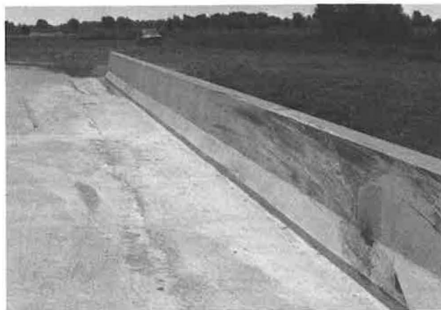
FIGURE 26 Thirty-two-in. F-shape after Test 7069-4.
