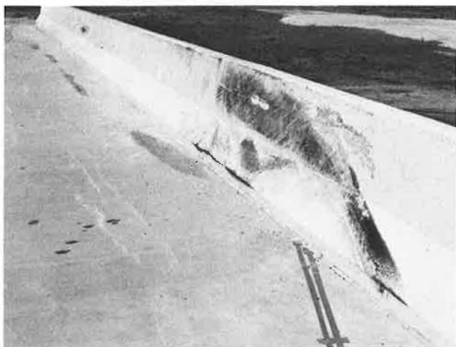
FIGURE 35 Thirty-two-in. New Jersey safety shape railing after Test 7069-12.
