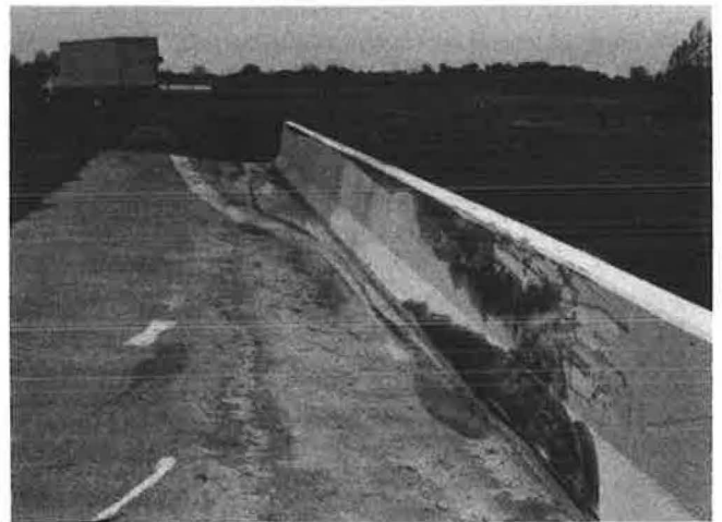
FIGURE 29 Thirty-two-in. F-shape after Test 7069-11.
