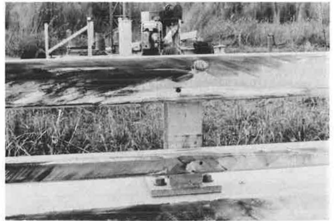
FIGURE 9 Damage to railing at Post 6.
