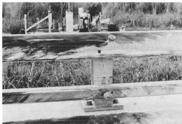
FIGURE 9 Damage to railing at Post 6.
