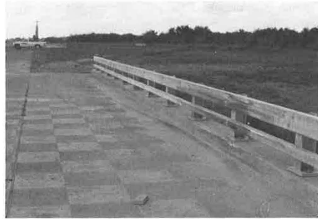
FIGURE 6 After-test photograph at railing in Test 7069-2.
