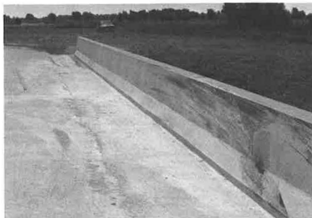
FIGURE 26 Thirty-two-in. F-shape after Test 7069-4.
