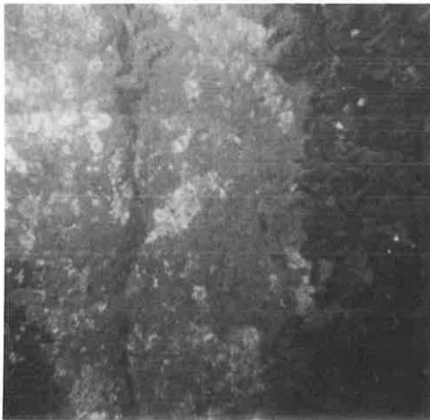
FIGURE 16 Two views of underwater cracks.
