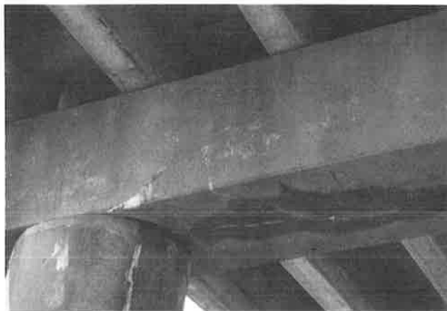
FIGURE 3 Cap with map cracking.
