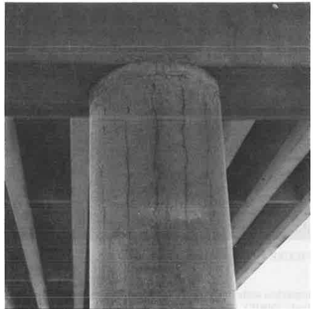
FIGURE 4 Pile with typical cracks.
