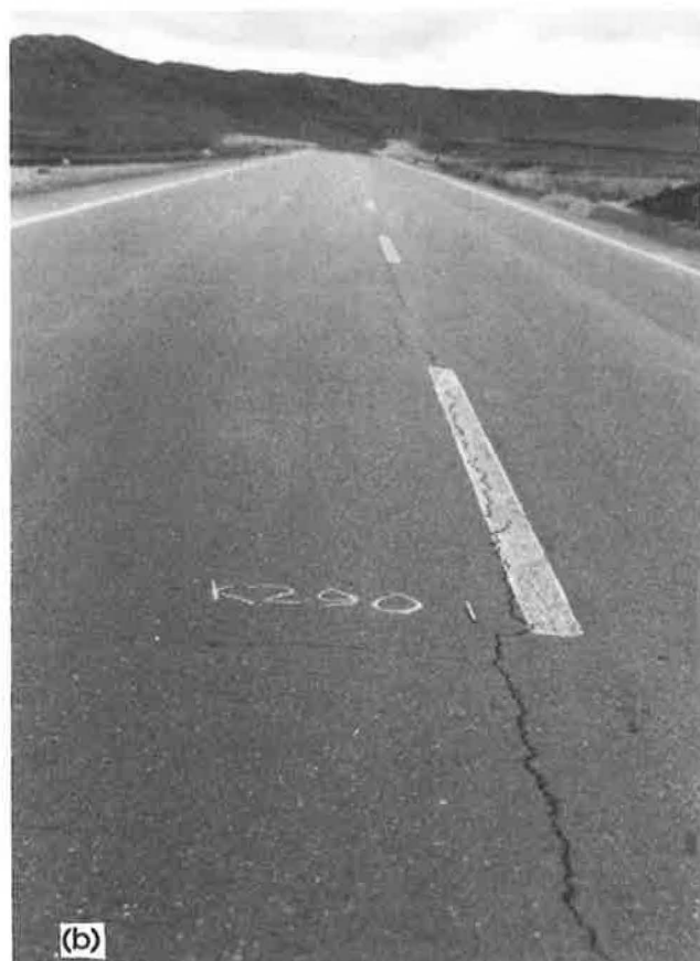
FIGURE 3 a, Typical longitudinal cracking; b, typical longitudinal joint cracking.
