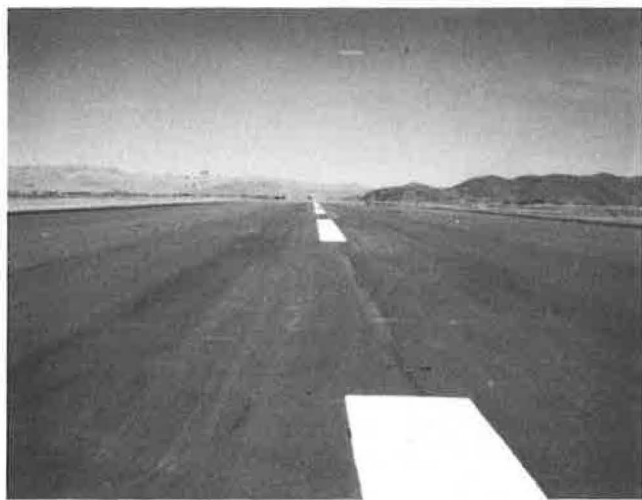
FIGURE 7 AC surface condition—Juliaca Airport at 3,890 MASL.
