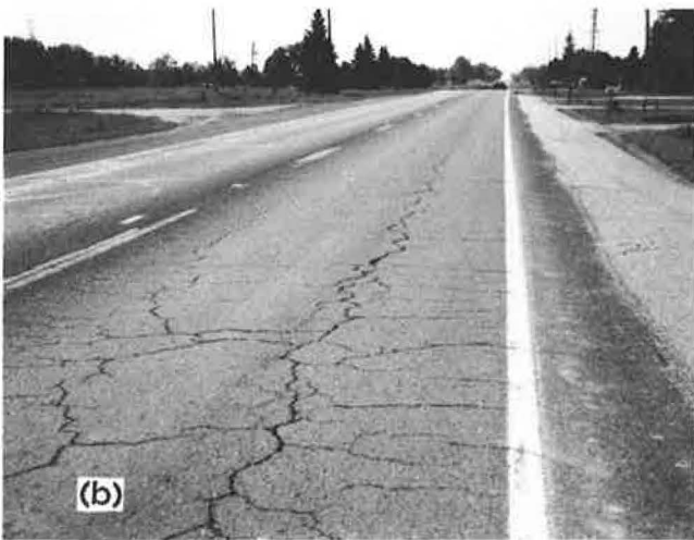
FIGURE 1 Cracking pattern observed on US-6, SR-55, and I-80/90: a, top view; b, longitudinal view.
