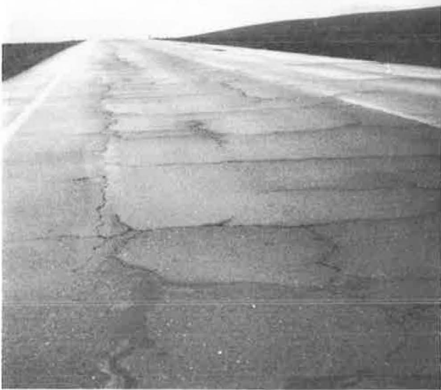
FIGURE 5 Typical pavement cracking, 2 years after completion of construction.
