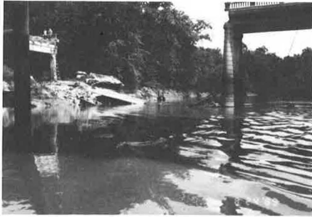
FIGURE 6 Span 79 debris removed.
