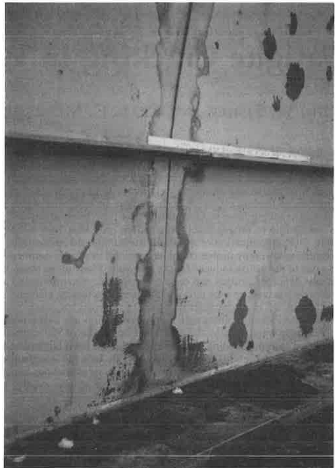
FIGURE 3 Crack originating from groove weld in longitudinal stiffener.
