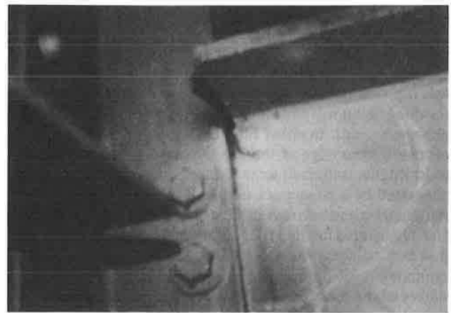
FIGURE 7 Fatigue crack in floorbeam web at end of welded flange.
