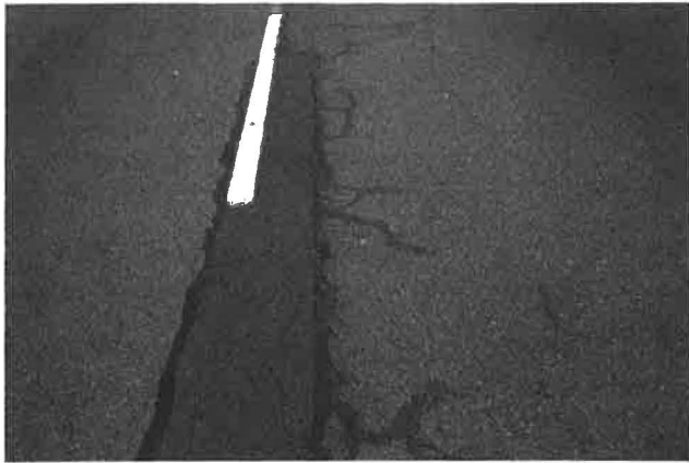
FIGURE 1 Typical longitudinal joint distress and repair.
