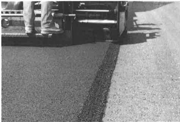
FIGURE 8 Initial unconfined wedge edge.
