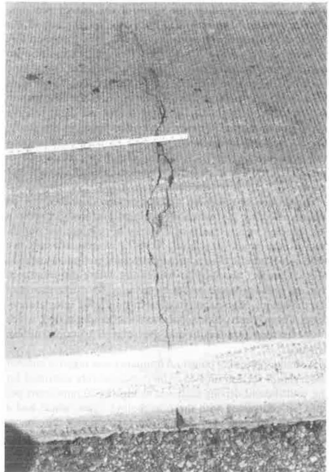
FIGURE 4 Type 1 spalling, I-39SB.
