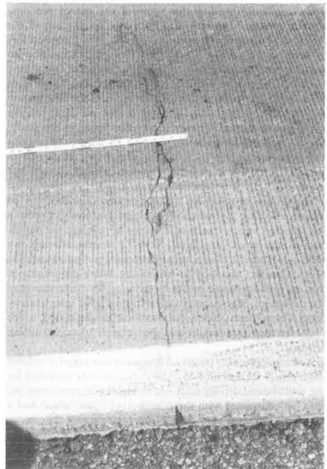
FIGURE 4 Type 1 spalling, I-39SB.
