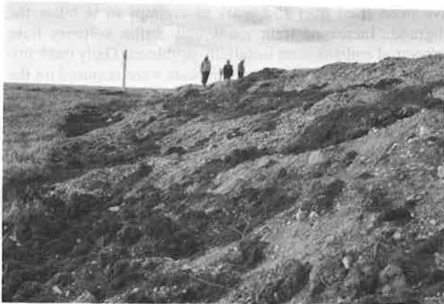
FIGURE 2 Photograph of failures at the site.
