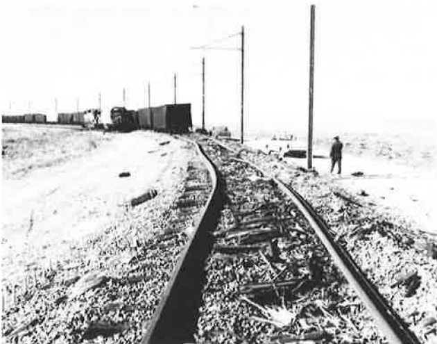
FIGURE 19 Track condition after derailment.
