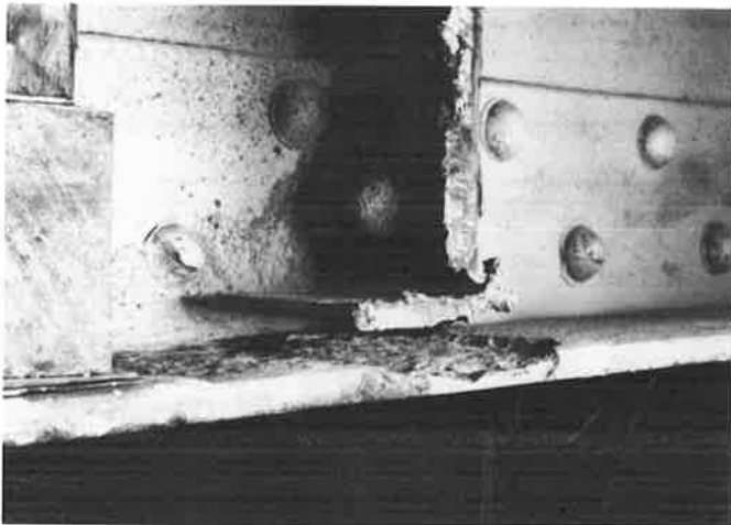
Figure 4 Corrosion Notched Flange Angle Below Diaphragm Where Dirt and Debris Accumulates
