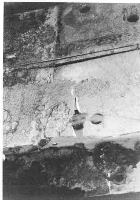
Figure 18 Crack in Flange of Hanger No. 1
