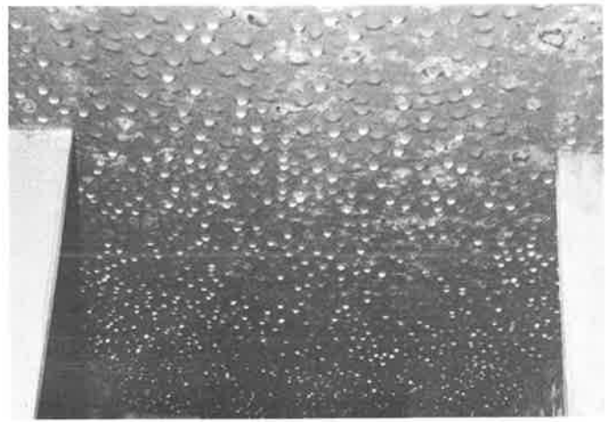
Figure 21. Condensation on Inside of Box Cap Member
