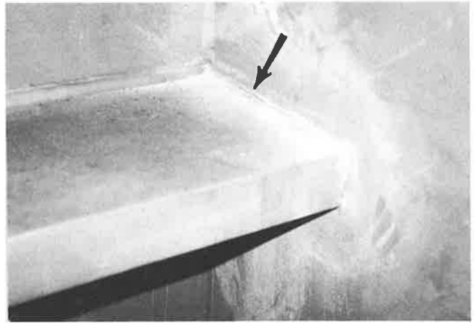
Figure 12. Crack in Seal Weld on Inside Face of Web of Box Cap Member
