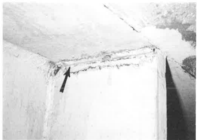
Figure 15. Crack in Weld Between Vertical Stiffener and Cap Upper Flange of Girder "T" Type Pier.
