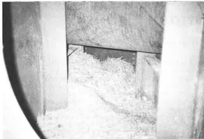
Figure 24. Nesting Material Inside Box Cap Member
