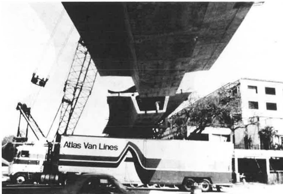
Figure 5. Biloxi, I-110. Balanced-cantilever construction over U.S. 90. Lane closures were made only as segments directly above were placed.
