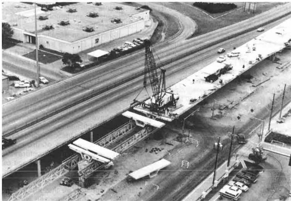
Figure 8. San Antonio "Y". Erection in the span-by-span method from above. Segments are delivered over the completed bridge. A deck mounted crane places segments on the erection trusses.
