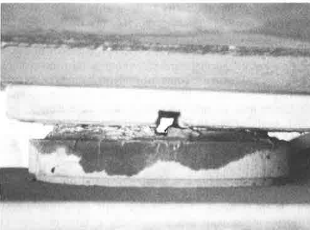
FIGURE 11 Misaligned guideway in a pot bearing due to transverse movement
