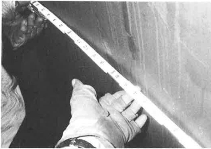
Figure 17. Cap Web Bowed at Web Splice Weld
