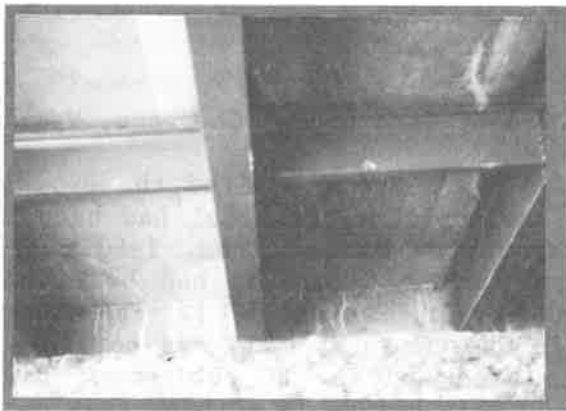
Figure 17. Diagonal cracking in bottom at end of isotropic deck.
