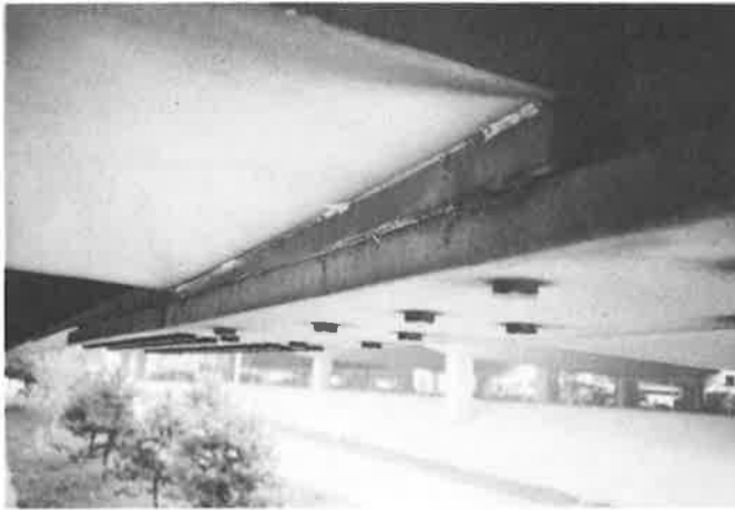
Figure 4. Fill Plate Between Cap and Girder Lower Flange is Stitch Welded to the Cap Lower Flange
