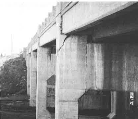
FIGURE 6 Minor spalling of concrete at piers due to transverse thermal movement
