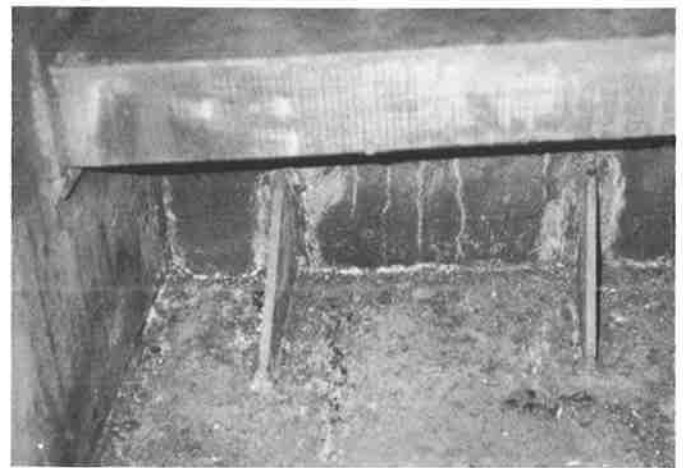
Figure 9. Diaphragm Stiffener Inside Box Cap Member is Welded to the Cap Lower Flange
