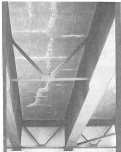
Figure 15. Bottom deck cracking at end.
