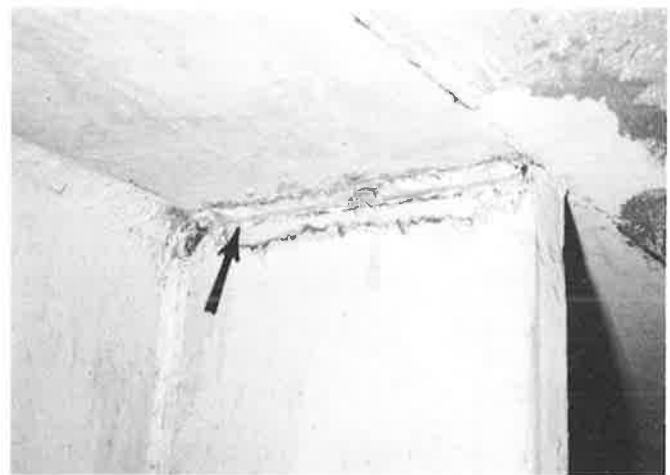
Figure 15. Crack in Weld Between Vertical Stiffener and Cap Upper Flange of Girder "T" Type Pier.
