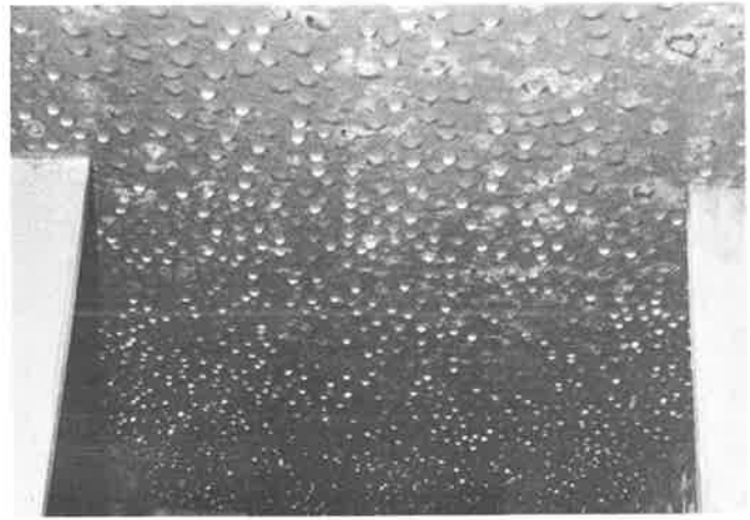
Figure 21. Condensation on Inside of Box Cap Member
