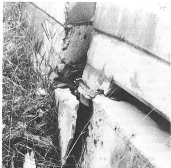
FIGURE 7 Misalignment of curb due to transverse movement of skew bridge
