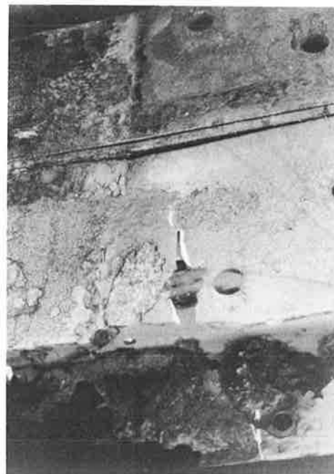
Figure 18 Crack in Flange of Hanger No. 1
