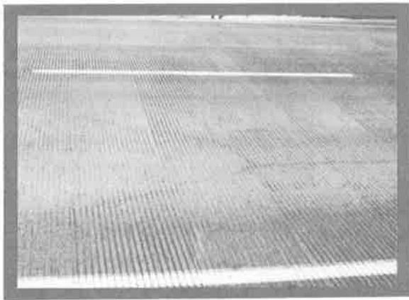
Figure 14. Top deck cracking at end.
