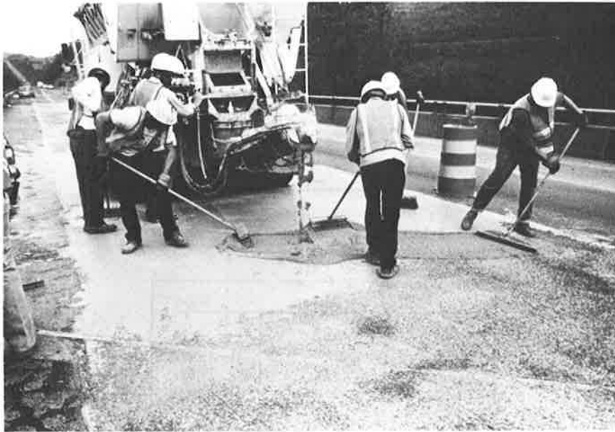
FIGURE 4 A latex modified slag slurry overlay is here applied to a bridge deck to increase the skid resistance. Brooms should be used to brush the slurry into the shot-blasted surface and the slurry should be struck off and pulled forward with gage rakes set to provide a 3/16 in to 1/4 in thick slurry. For increased skid resistance slag should be broadcast onto the struck off surface, and a liquid curing material should be applied to prevent the evaporation of water. The slurry can be opened to traffic in two to three days.
