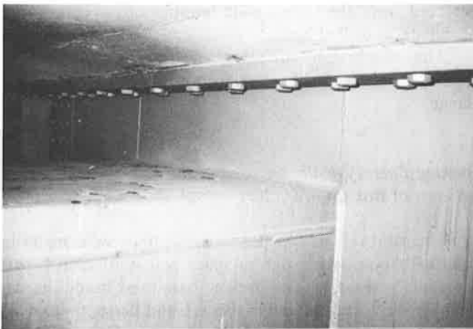
Figure 5. Girder Upper Flange and Web are Continuous Over the Cap Upper Flange.
