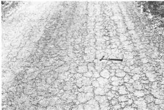
FIGURE 1 Alligator cracking and raveling without distortion indicating bitumen aging.
