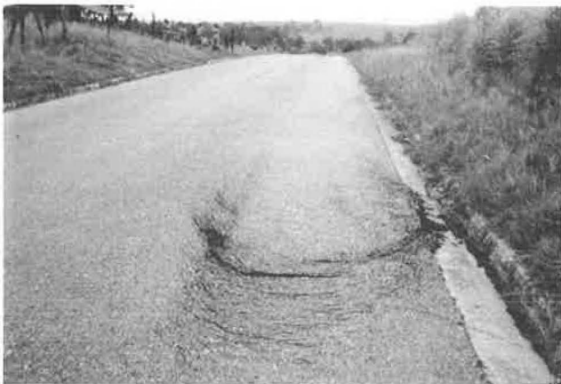
FIGURE 10 Peeling and crescent-shaped cracks, National Road 1, Zaire: the tack coat binding the soil-cement base to the wearing course was sheared by driving up heavy vehicles.
