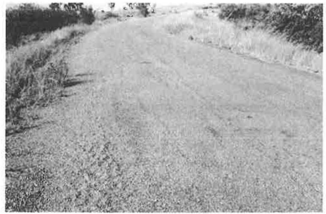
FIGURE 11 Longitudinal cracks and settlements of a poorly compacted embankment between Malaimbandy and Miandrivazo, National Road 35, Madagascar.
