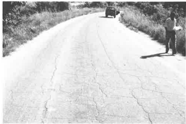
FIGURE 7 Block cracking of a soil-cement base: Kilometer 89, National Road 6, Madagascar.
