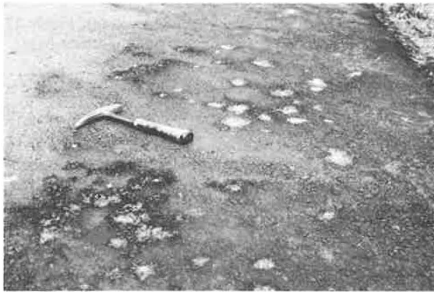
FIGURE 19 Cracked blisters and rust staining along the shoulders of National Road 12, Kilometer 133, between Manakara and Farafangana, Madagascar.
