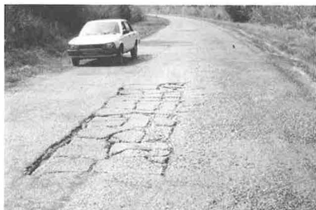
FIGURE 8 Block cracking resulting from tensile failure of a soil-cement pavement: Masiaka Road, Sierra Leone, 1982, before rehabilitation.
