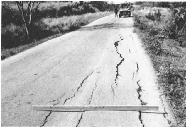
FIGURE 14 Longitudinal cracks and collapsed voids (National Road 6, between Port Bergé and Antsohihy, Madagascar).
