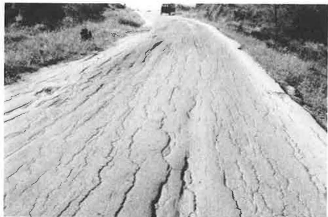
FIGURE 16 Longitudinal cracks, settlements, and undulations typical of expansive subgrade soils (National Road 6, between Mampikony and Port Bergé, Madagascar); the car is parked on a stable subgrade section.
