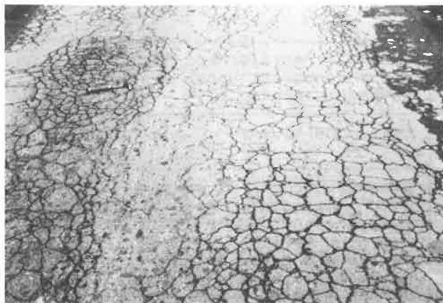
FIGURE 2 Alligator cracking of a depressed area indicating low bearing capacity of pavement structure.
