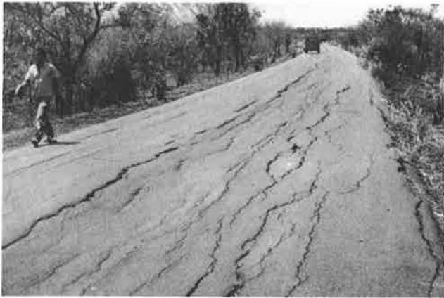
FIGURE 13 Well-developed distress pattern typical of expansive subgrade soils; longitudinal cracks and differential settlements (National Road 6, Kilometer 225, Madagascar).
