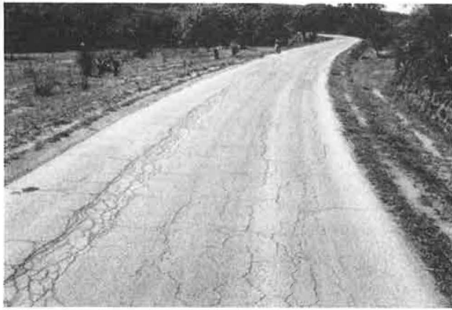
FIGURE 9 Two different families of block cracking, Kilometer 0+200, National Road 32, Madagascar: widely spaced shrinkage cracks, and narrow tensile failure block cracks associated with ruts.
