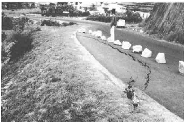
FIGURE 6 Longitudinal curved crack and settlement resulting from embankment slope slide, National Road 7, in the vicinity of Ambatolampy, Madagascar.
