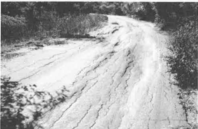
FIGURE 15 Longitudinal cracks, settlements, and collapsed voids (National Road 6, between Mampikony and Port Bergé, Madagascar).
