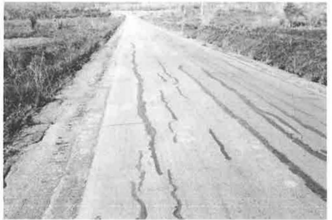
FIGURE 12 Longitudinal cracks developed during the first dry season in sections of National Road 3, Kilometer 73, Benin, where the embankment had been constructed with expansive clays (lama depression). The cracks were carefully sealed but reopened during the next dry season.
