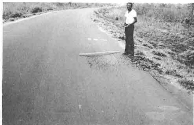
FIGURE 17 Local shearing of a soft sandstone gravel, Kilometer 3 from Pobe, National Road 3, between Porto Novo and Pobe, Benin, 1985, before rehabilitation.
