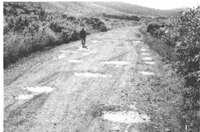
FIGURE 9 Potholing of a well-graded crushed-stone pavement, National Road 5A, Madagascar.
