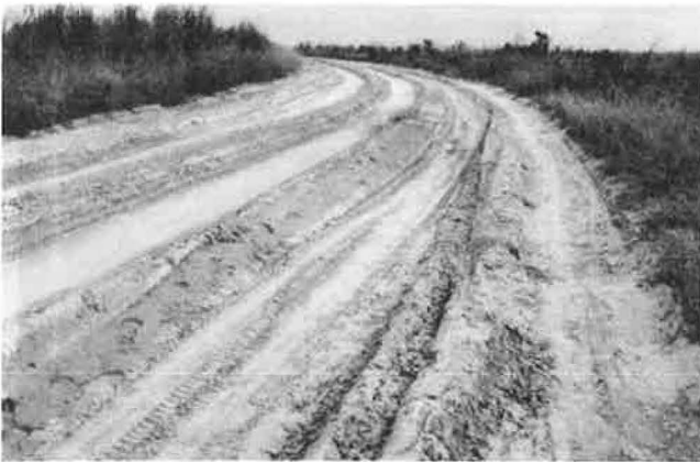
FIGURE 11 Rainy season rutting of a recently rehabilitated earth road, Bandundu province, Zaire.
