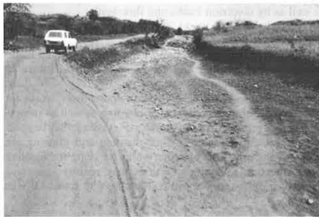
FIGURE 15 A poorly drained entrenched section of an earth road resulting from periodic maintenance by scraping has been deviated by traffic.
