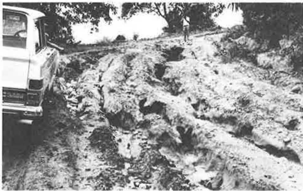
FIGURE 3 Erosion on steep gradient.
