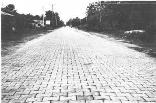
FIGURE 6 Concrete blocks after 18 months' trafficking.
