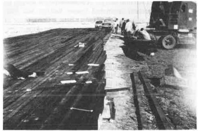
FIGURE 9 Continuous 150-ft stressed deck being readied to be launched or skidded onto the steel stringers.
