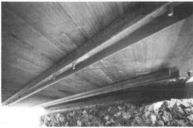
FIGURE 5 Steel distributor beams.
