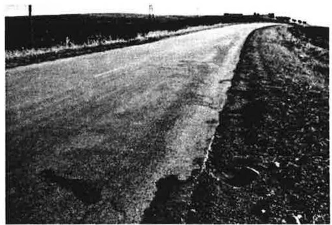
FIGURE 3 Edge settlement and water outflow through longitudinal cracks.
