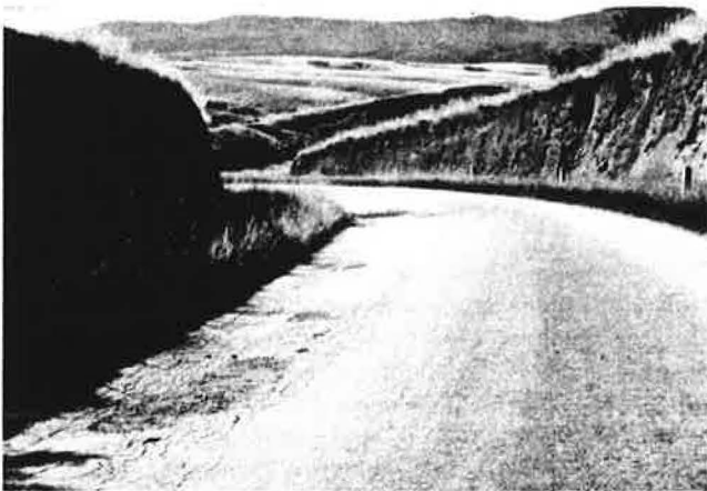
FIGURE 2 Longitudinal cracks and settlements along the shoulder, typical of poorly drained pavement.
