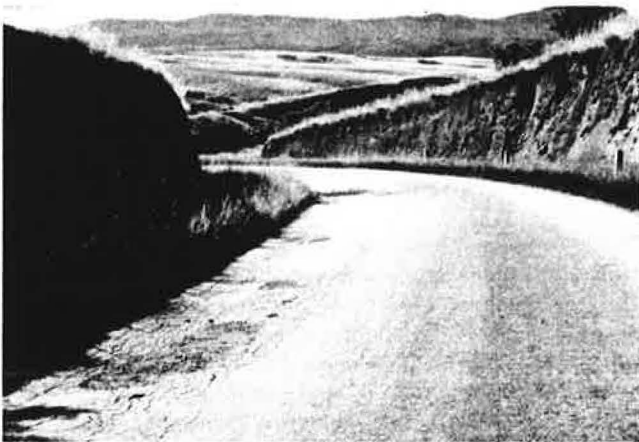
FIGURE 2 Longitudinal cracks and settlements along the shoulder, typical of poorly drained pavement.
