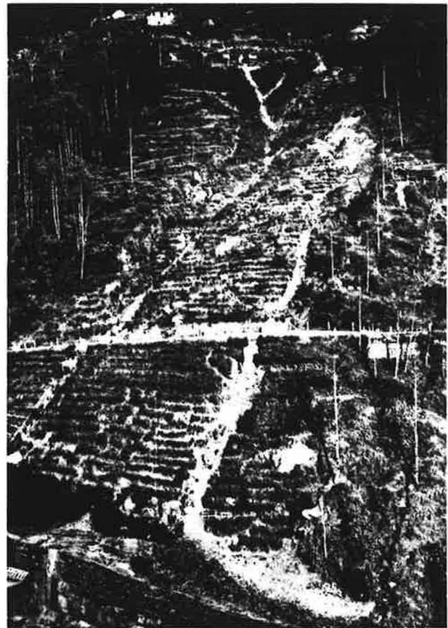
FIGURE 7 Stabilized slide at Charnawati left bank, Km 45.1. Two main drains crossing the road are supported by the gabion guidewall at the river.
