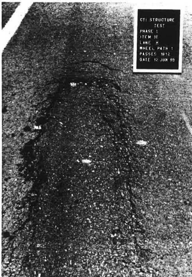
FIGURE 7 High-pressure lane, Section 10, shoving after 1,812 passes.
