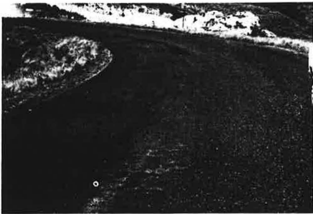
FIGURE 1 Alligator cracking, loss of fines, and springs along the centerline of an embankment section at Kilometer 21+700, National Road 12.
