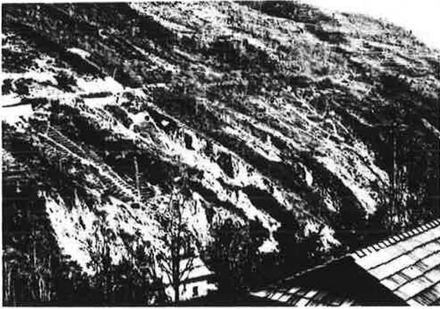
FIGURE 8 General view of slides, Km 45.4 to 46.0. Drainage and biotechnical measures can be seen in the upper parts of the slides.
