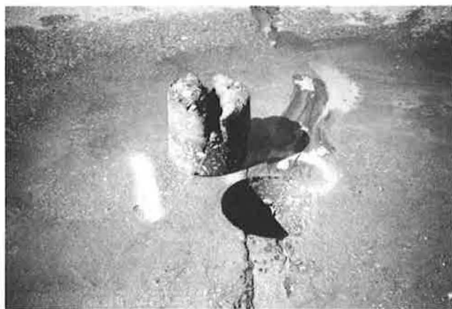
FIGURE 8 Core of transverse cracks in Section 1.
