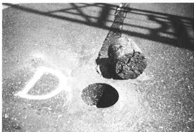
FIGURE 6 Core of transverse crack taken from high side of superelevated curve in Section 2.
