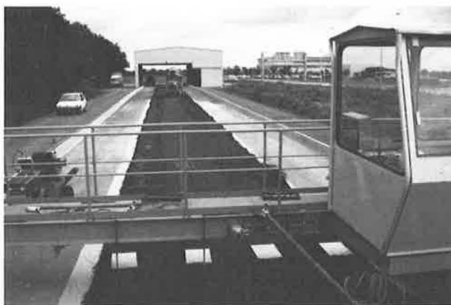
FIGURE 2 Spreading of rolled asphalt on the LCPC test track at Nantes and recording of the level of the course by the measuring carriage.
