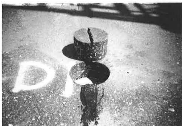
FIGURE 7 Core of transverse crack taken from low side of superelevated curve in Section 2.
