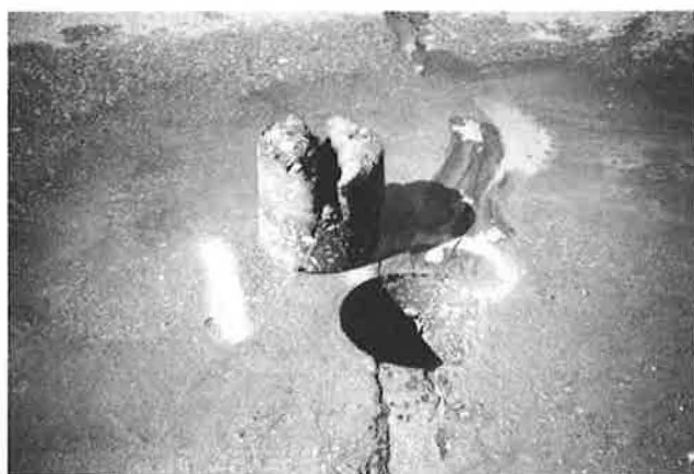
FIGURE 8 Core of transverse cracks in Section 1.
