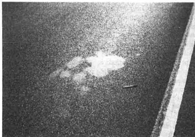
FIGURE 3 Typical localized bleeding area, northbound lanes of I-55 near Collinsville, Ill.
