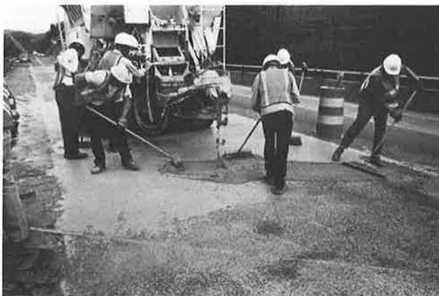
FIGURE 1 A latex-modified slag slurry overlay is applied to a bridge deck to increase the skid resistance.
