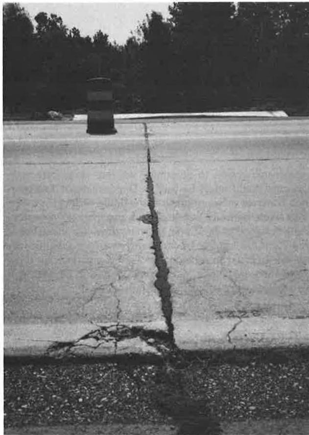
FIGURE 1 Typical map cracking caused by AAR, I-295, Burlington County, New Jersey.
