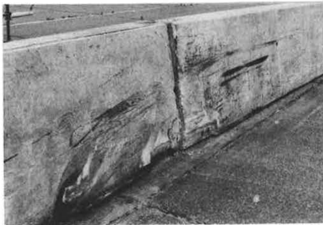
FIGURE 14 Single-slope barrier after Test 4.
