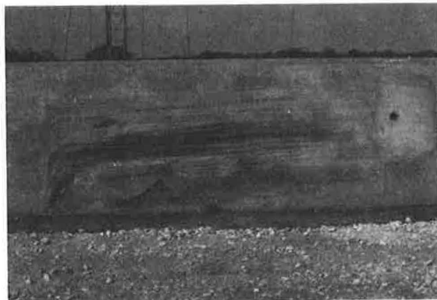
FIGURE 8 Single-slope barrier after Test 2.
