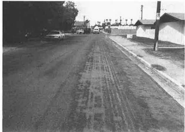
FIGURE 3 Chip loss on street edge.
