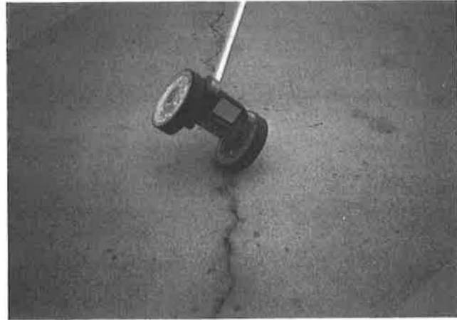
FIGURE 5 Measurement of crack length using edge of roller-tape.
