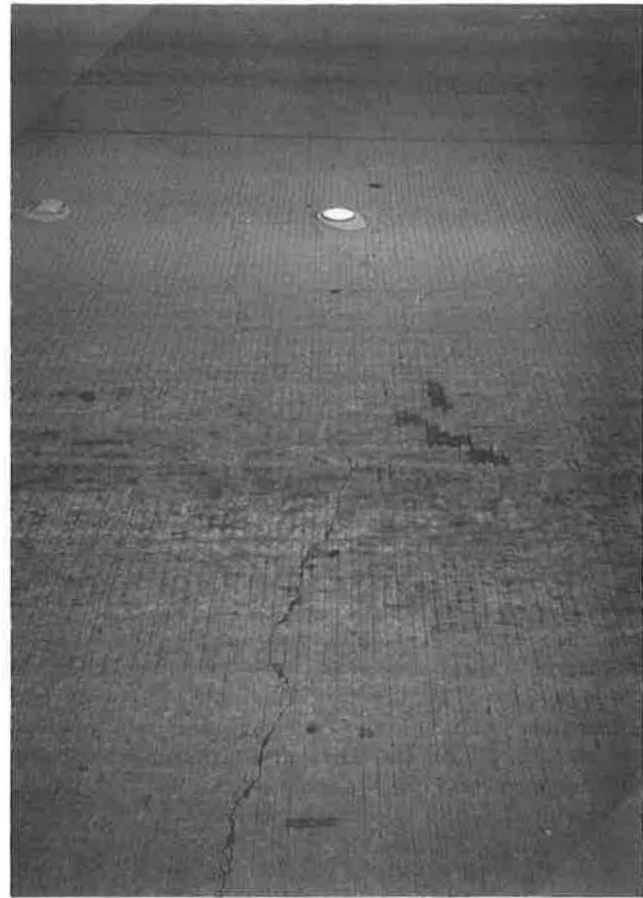
FIGURE 11 Crack with RI value of 1.8 ( R = 7.3 percent and N = 2 ).
