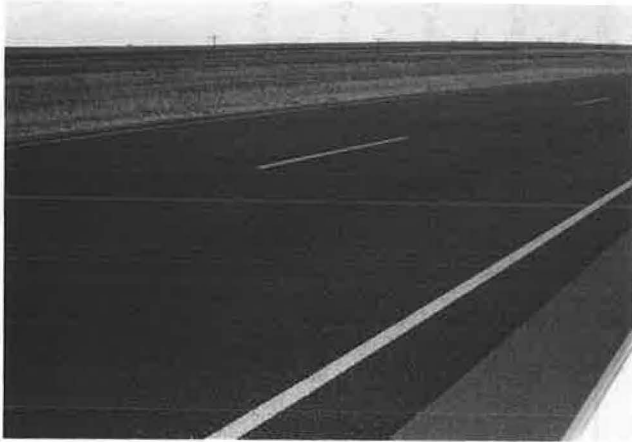
FIGURE 2 Condition of the roadway on Project IR-040-5(40)282 in the control section without cracking and seating or paving fabric. Note the two transverse cracks spaced approximately 40 ft apart.
