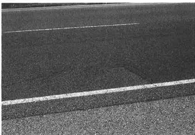
FIGURE 4 Reflection cracking, better described as reflective corner break, on Project IR-040-5(42)300.
