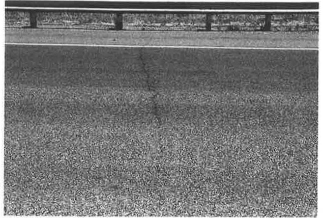
FIGURE 3 Reflection cracking evident in a section near MP 300.5 on Project IR-040-5(42)300.
