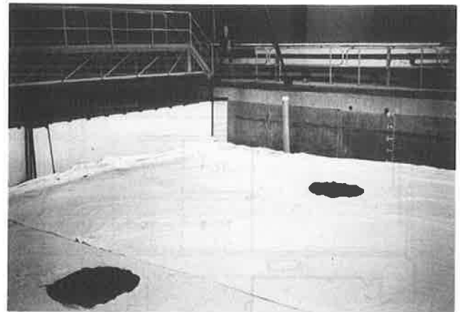
FIGURE 6 Geotextile being installed and the 1.2-m-diameter hole in the geotextile around the instrumentation in Test Cells 10 and 11.
