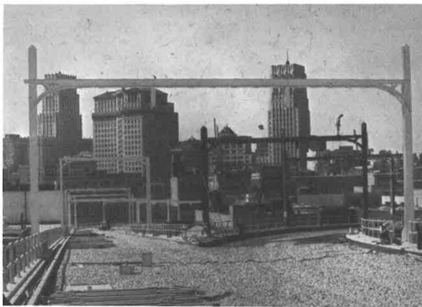
FIGURE 6 Terminal viaduct under construction. Note gravel track ballast and overhead trolley wire support frame. Trains proceeded counterclockwise at the gore. Source: Caltrans.
