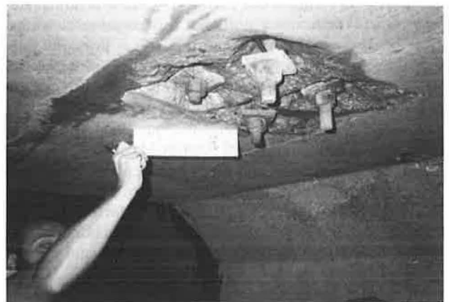
FIGURE 4 Spalling of concrete around guardrail bolt holes.
