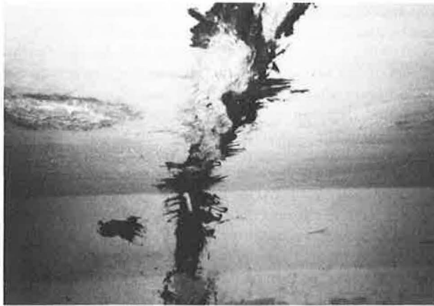
FIGURE 5 Serious joint leakage, salt deposits, and corrosion.
