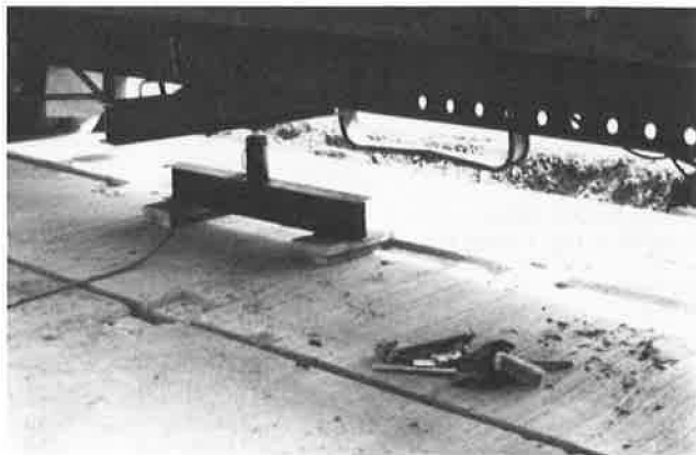
FIGURE 5 Load was applied by hydraulic jack in 7,800-lb increments to a maximum load of 31,200 lb. Load was distributed on the 10- x 20-in. bearing areas at 4-ft centers to simulate truck wheel bearing areas. The 31,200-lb load is equivalent to the ASTM C850 Interstate alternate axle loading.
