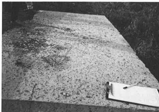
FIGURE 6 Spalling on top surface of box culvert.
