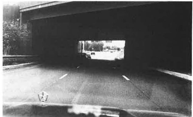
FIGURE 4 Bridge span blockage.
