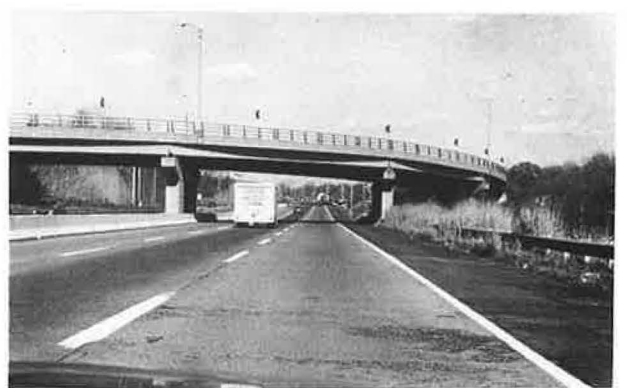
FIGURE 5 Bridge pier blockage.
